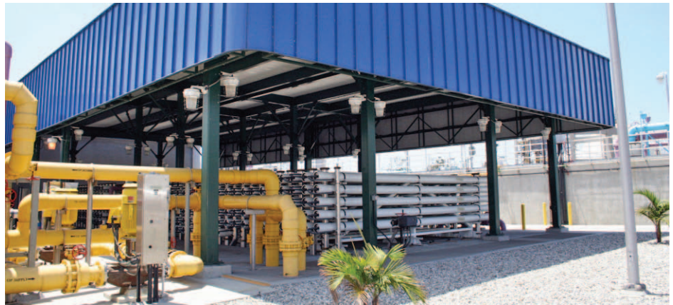
AWPF at TIWRP producing highly purified water
