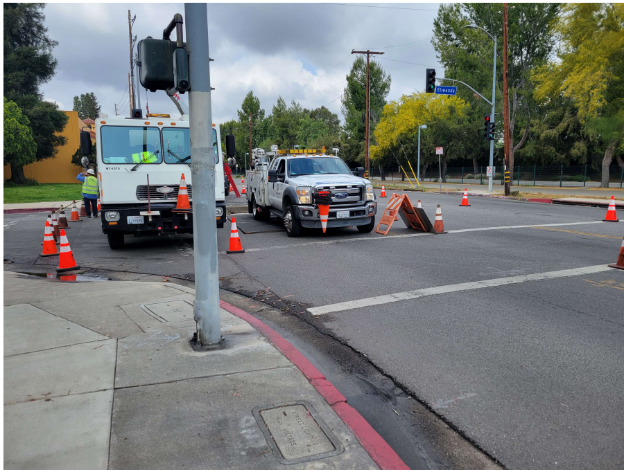
Plate 8: Overview of an underground section being repaired at West Oxnard Street and Etiwanda Avenue, view to west, April 28, 2022
