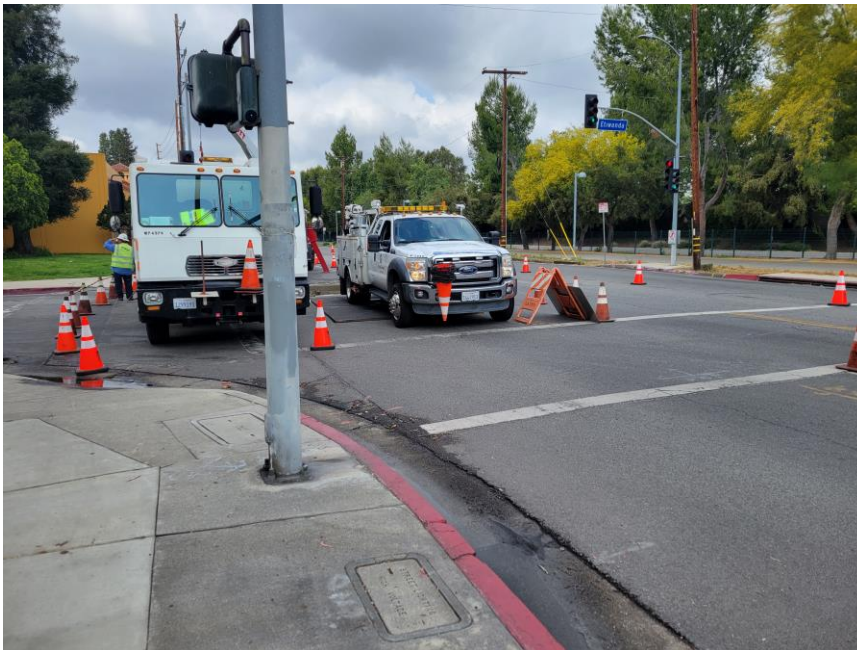
Photograph 2. Overview of an underground section being repaired at West Oxnard Street and Etiwanda Avenue, view to west, April 28, 2022
