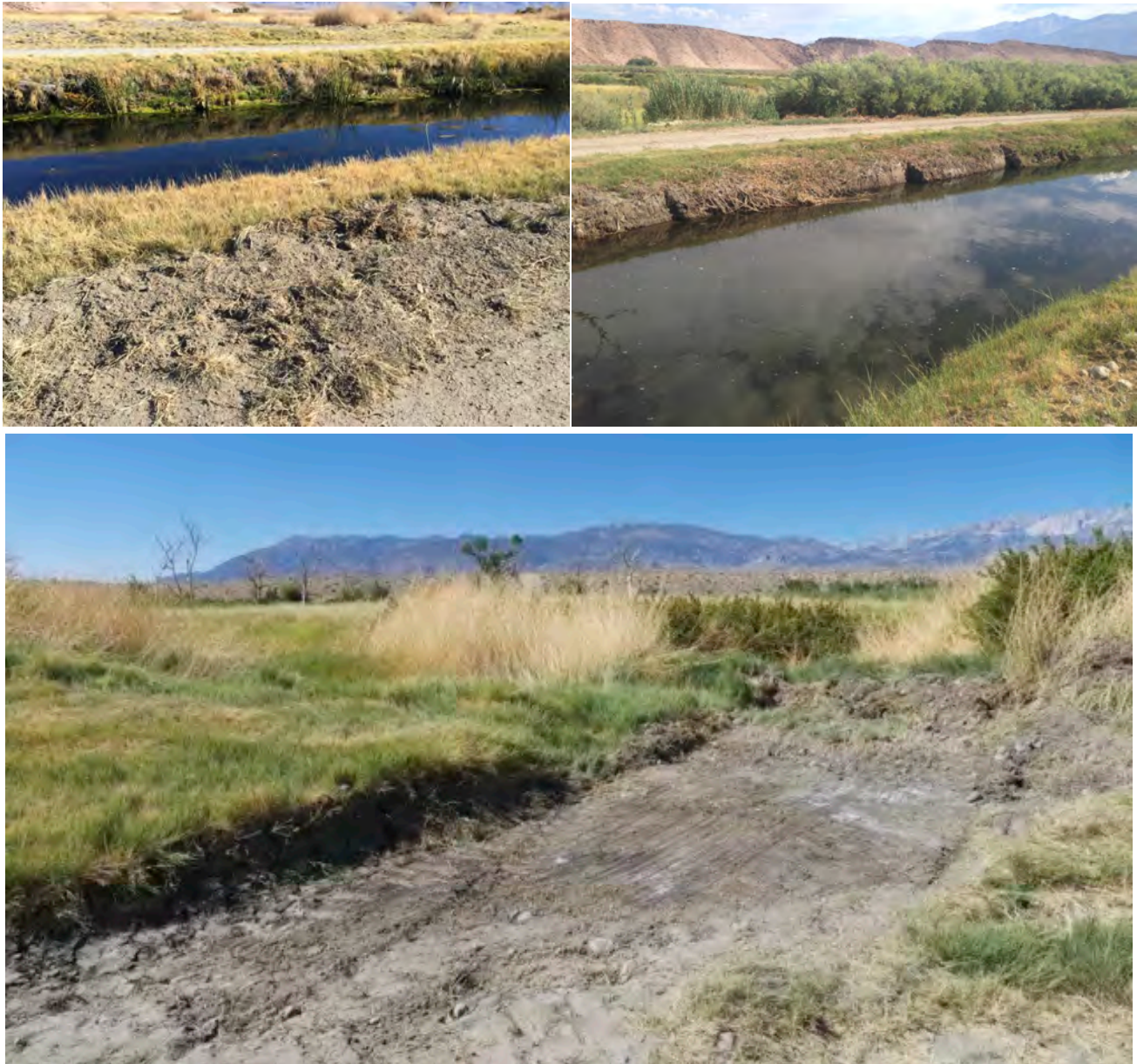
Upper left: Meadow vegetation mowed to dirt level on bank of Bishop Creek canal (photo taken November 9, 2014). Upper right: Vegetation and portions of far bank have been graded and/or chopped away during routine maintenance (photo taken July 17, 2014). Bottom: Meadow scraped and graded away during routine maintenance (photo taken November 9, 2014).
