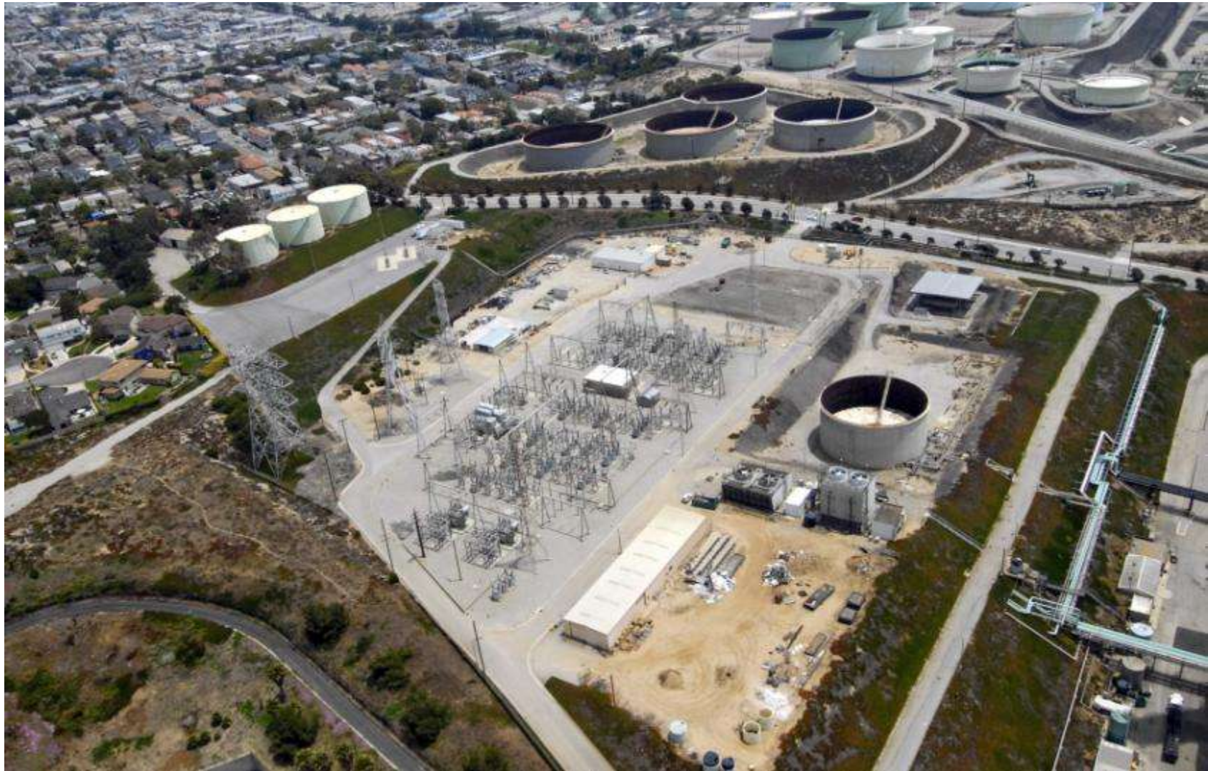
FIGURE 3.3-4. SITE FACILITIES – SWITCHING YARD, WATER CONDITIONING TANKS, AND ABANDONED FUEL OIL STORAGE TANKS
