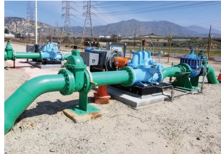
The new pumping units 1 and 6 at the Penstock Pump Station in Granada Hills help increase reliability, redundancy and capacity of water supply.
