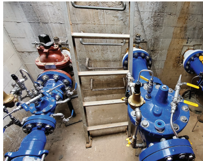
The Villa Woods Regulator Station in the Pacific Palisades area serves as a supply and pressure regulating station.
