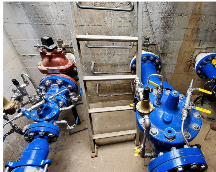
The Villa Woods Regulator Station in the Pacific Palisades area serves as a supply and pressure regulating station.
