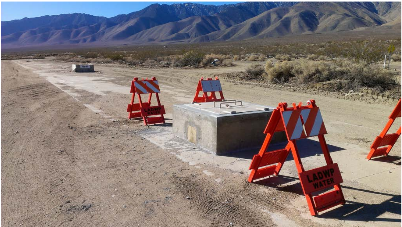
Concrete access box atop the concrete cover for LAA1. Pipeline from well V817 will connect to this access box to deliver pumped well water.
