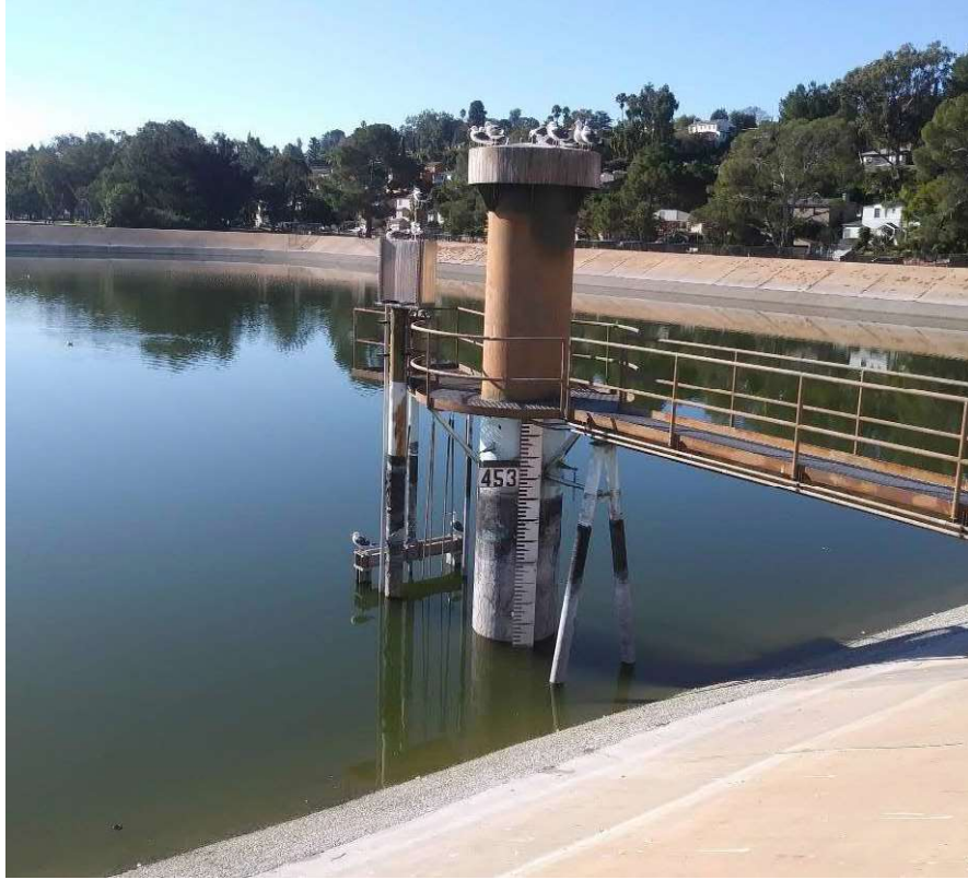
Photo 1. Southwest-facing view of the Ivanhoe Inlet Tower at the north end of Ivanhoe Reservoir.
