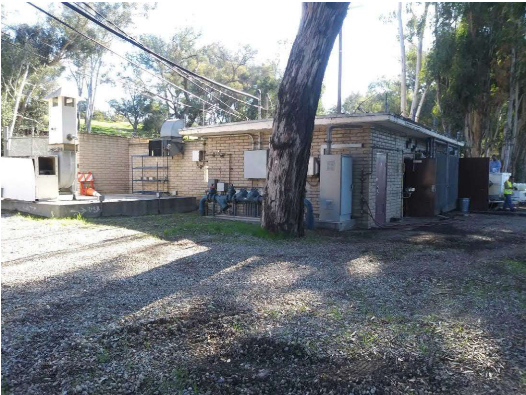
Photo 4. Southeast-facing view of the chlorination station on the east side of Silver Lake Reservoir, where the Air Blower Closure will be installed.
