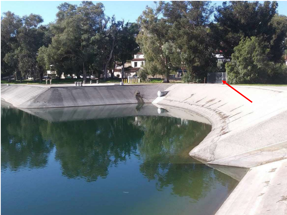
Photo 2. West-facing view of Gate 456 Structure (red arrow) at northwest corner of Silver Lake Reservoir.
