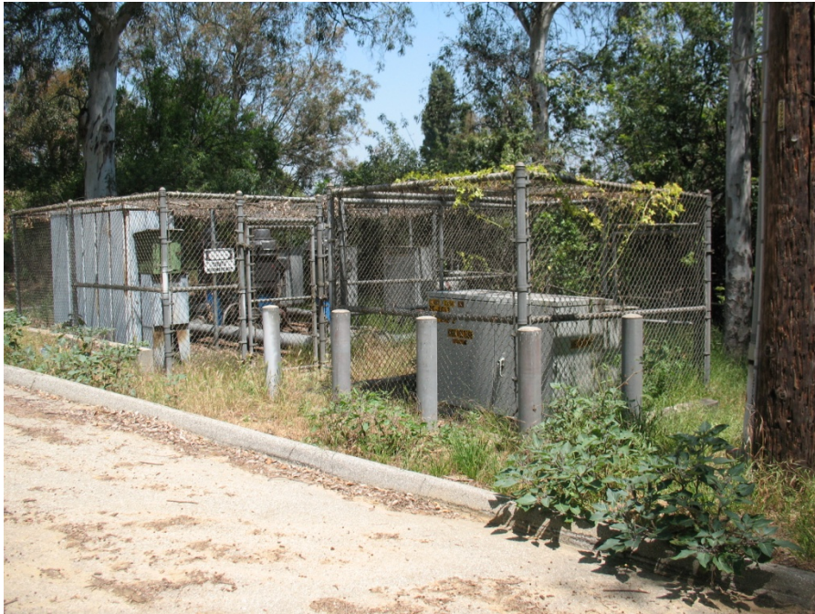
Photo 8. Existing electrical boxes and utilities are located immediately northwest of the proposed recycled water pumping station location. Photo facing north.
