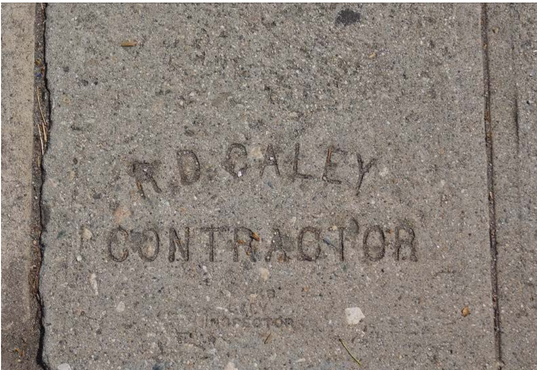
Figure 90. Sidewalk along Southbound Broadway between 18th and Washington, “R.D. CALEY CONTRACTOR,” View West
