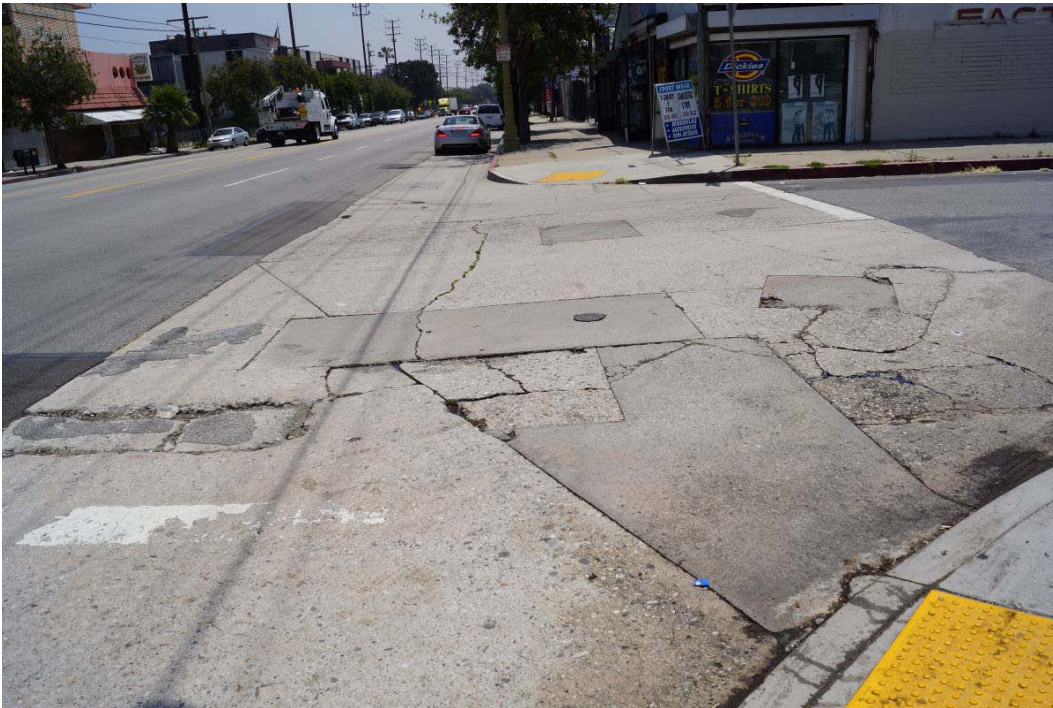
Figure 94. Disturbance to 1930 Olympic Boulevard Street Surface, View West
