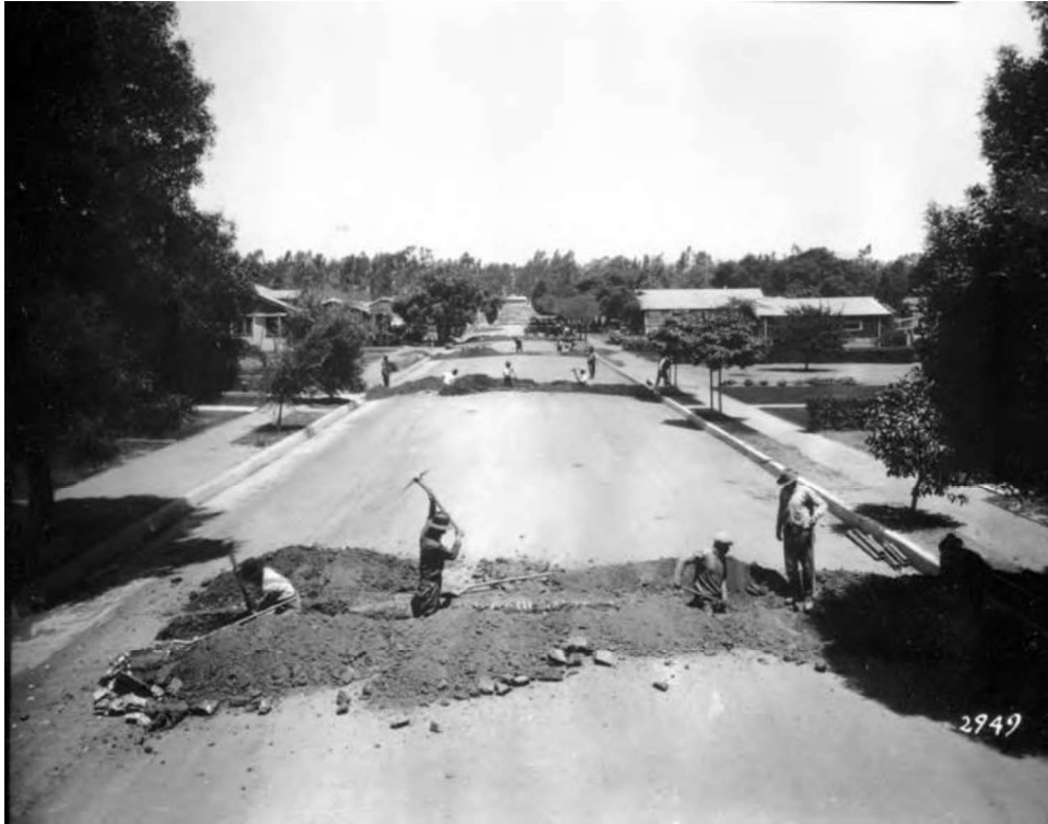
Figure 6. Trunk line construction, no date/location (DWP Photo Collection, Los Angeles Public Library)
