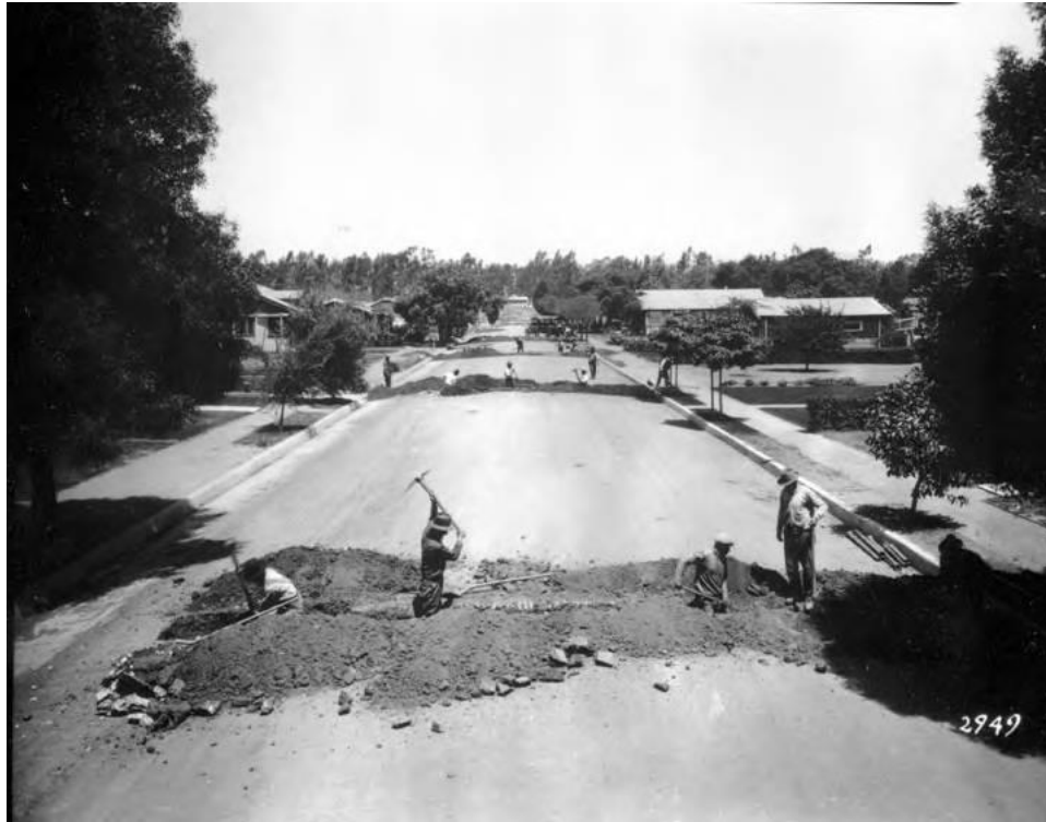
Figure 8. Trunk line construction, no date/location (DWP Photo Collection, Los Angeles Public Library)
