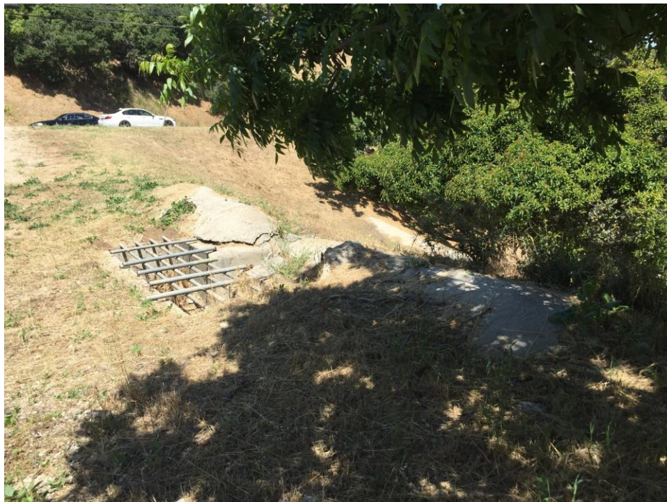
Figure 14. Flow Control Station Inlet Header and top runnel, looking southwest (IMG_3655)
