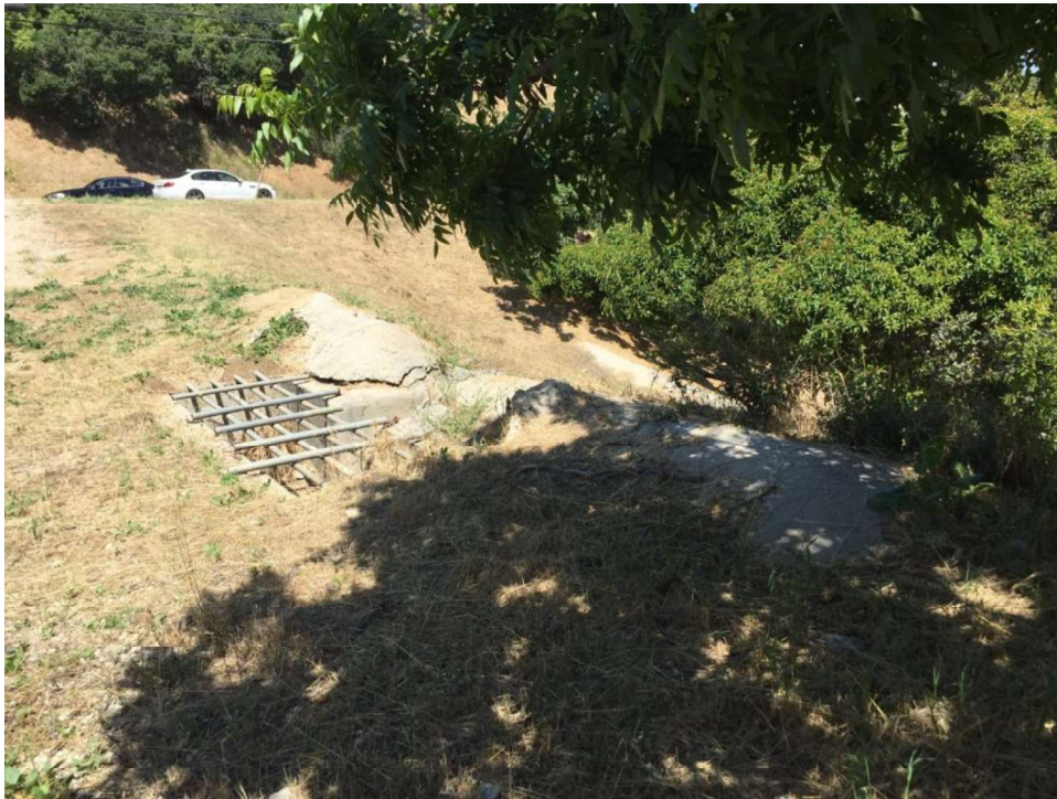
Figure 3. Flow Control Station Inlet Header and top runnel, looking southwest (IMG_3655)
