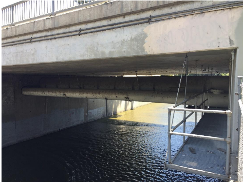
Figure 11. View of visible portion of City Trunk Line South segment pipe, in background behind smaller diameter pipe. View to east (IMG_3683)
