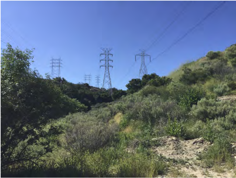
Southern portion of the alignment, where the alignment crosses open space areas in unincorporated Los Angeles County.
