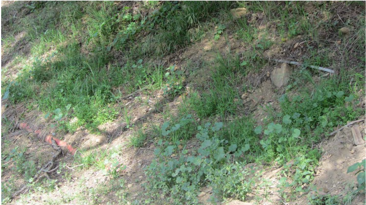
Figure 29. Exposed Water Pipes Adjacent to Fire Road, View North
