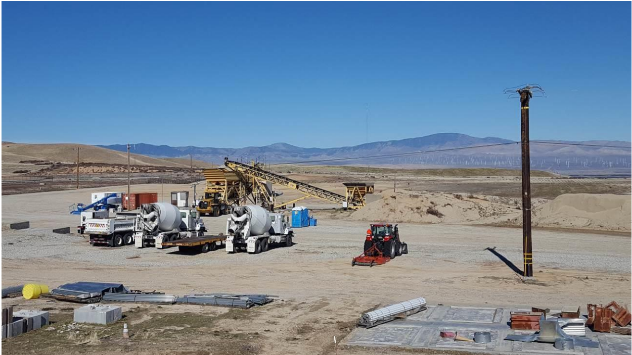
Photo 4: North-facing view of proposed staging and laydown area occurring south of the site for the proposed sedimentation plant (photo taken May 18, 2017).
