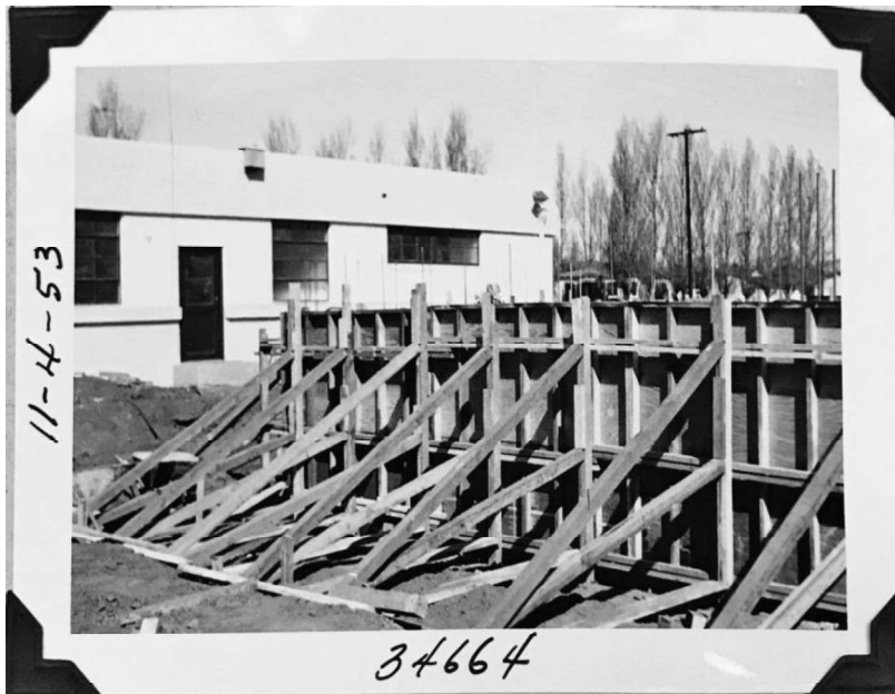
West Los Angeles Headquarters, Building 2 (warehouse), exterior form for west foundation wall; November 4, 1953 (LADWP No. 34664)
