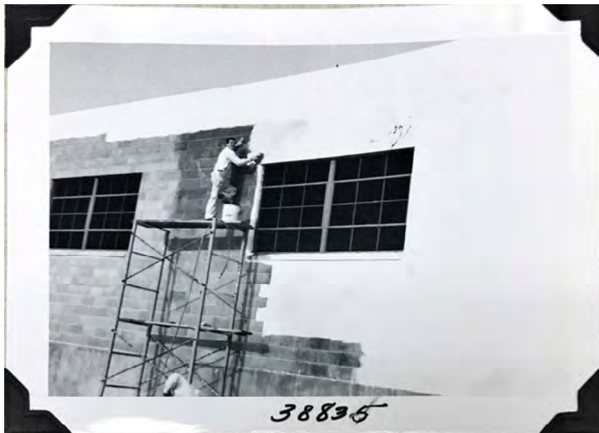
West Los Angeles Headquarters, Building 2 (warehouse), brushing on Wesco X-tite Coater on west wall; February 10, 1954 (LADWP No. 38835)
