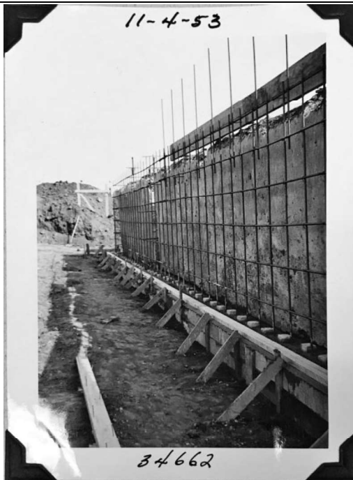
West Los Angeles Headquarters, Building 2 (warehouse), north end of fill showing footing and reinforced steel for foundation wall ; November 4, 1953 (LADWP No. 34662)
