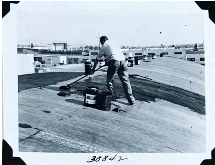
West Los Angeles Headquarters, Building 2 (warehouse), mopping roof with Pioneer C-13-C4 Asphalt emulsion (Pioneer); February 17, 1954 (LADWP No. 38842)
