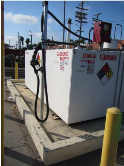
Photograph 29 – Photograph showing a gasoline AST and nozzle.
