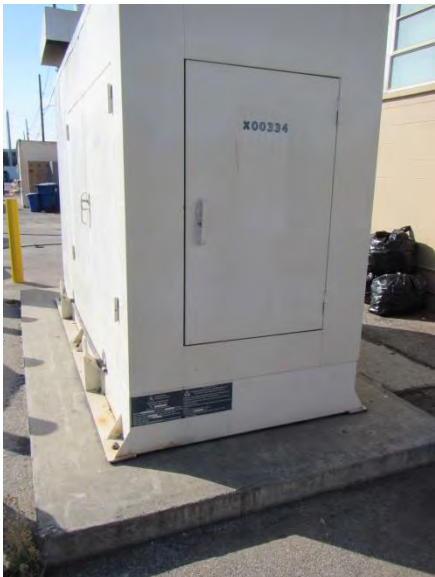
Photograph 31 – Diesel emergency generator located on the northwestern portion of the subject property.
