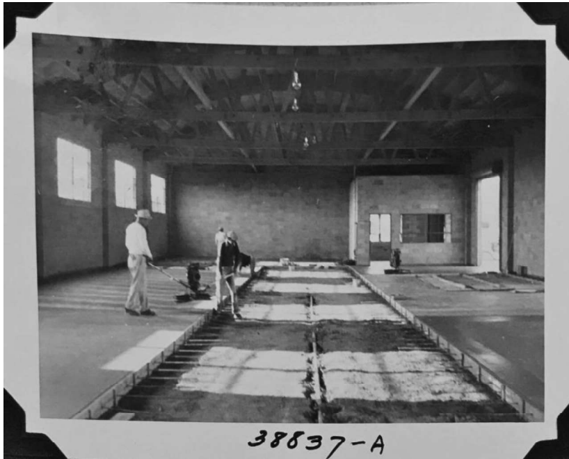
West Los Angeles Headquarters, Building 2 (warehouse), placing of floor slab; February 10, 1954 (LADWP No. 38837A)
