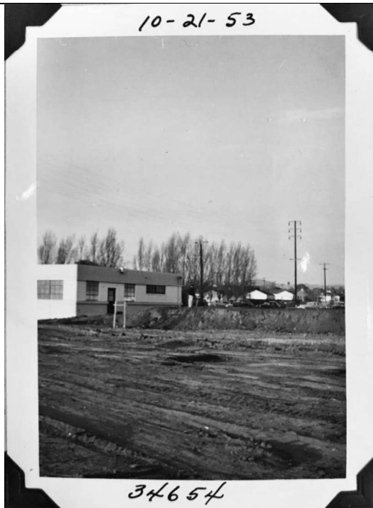
West Los Angeles Headquarters, Building 1 (locker room) in background, clearing foundation for Building 2 (warehouse); October 21, 1953 (LADWP No. 34654)
