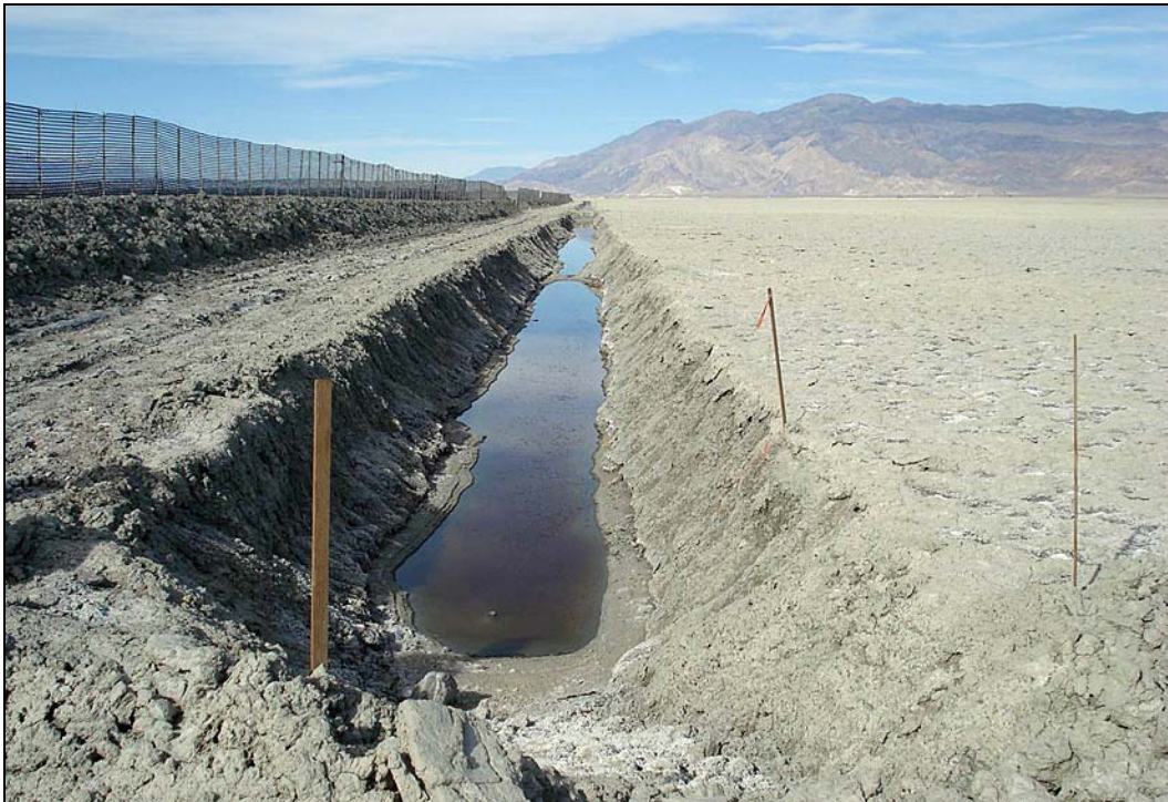
Looking north along moat on eastern border of cell T12-1 showing groundwater within the moat. (Photograph taken by EDAW on November 13, 2008)
