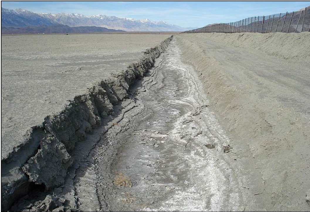
Looking north along moat on western border of cell T32-1 showing indicators of groundwater within moat. ( Photograph taken by EDAW on November 14, 2008 )
