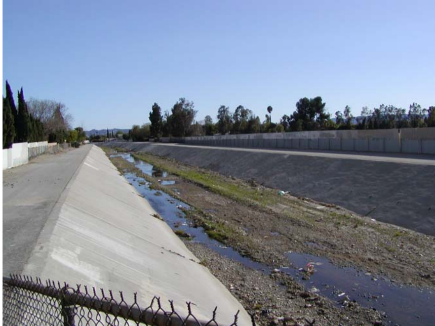
Pacoima Wash facing south from Roscoe Boulevard 0.5 mile east of Sepulveda Boulevard
