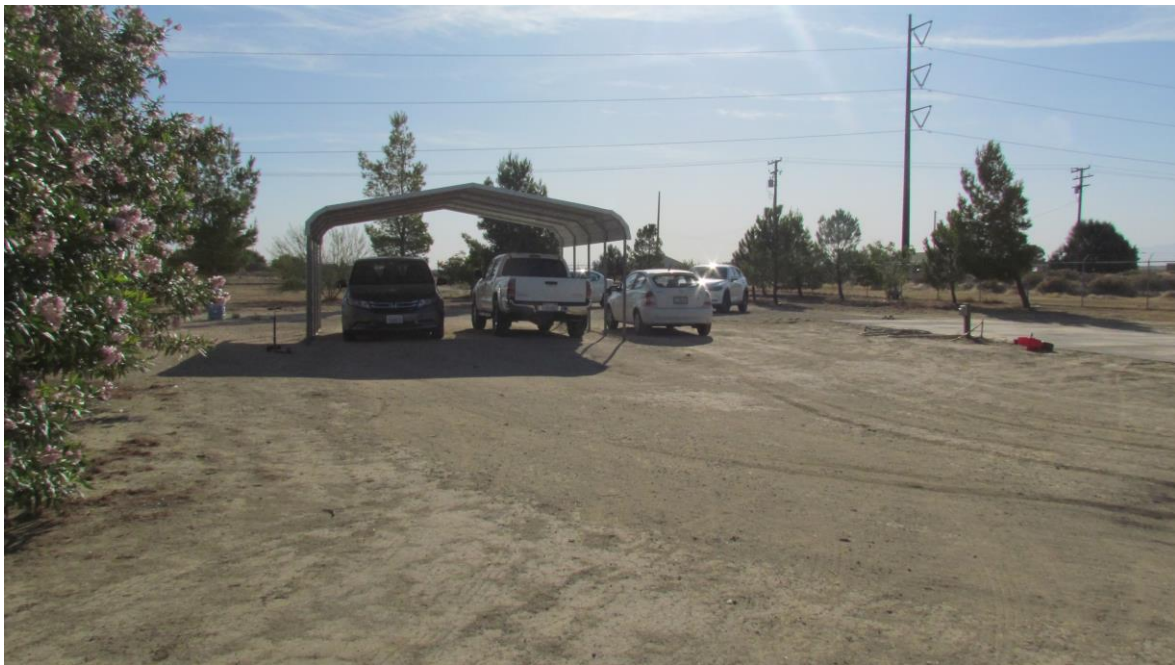
Photograph 8 - View facing east on residential property (2929 100 th Street West) that adjoins north of the Site. Pole-mounted transformers along eastern Site boundary are shown in background.
