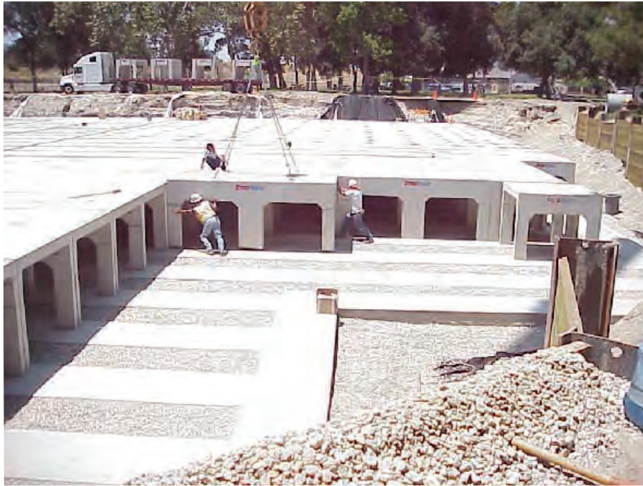
Sun Valley Park Infiltration Galleries
