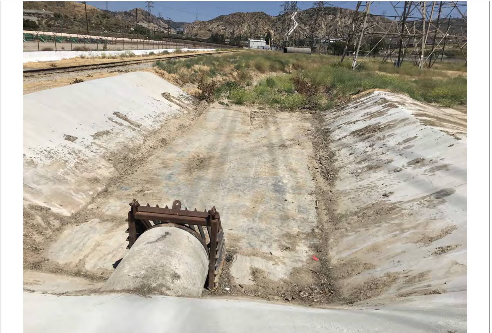
FIGURE 3C San Fernando Gate Drain LADWP Van Norman Complex
